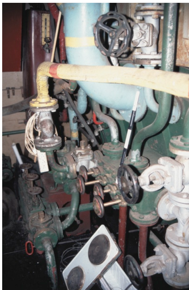
The condensing water controls.
